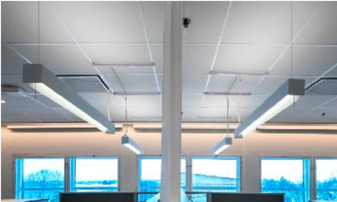
Schaeffler office refurbishment, Arlandastad, 2021 General and task lighting using pendant luminaire 'Plain' from Anell Ljus + Form
